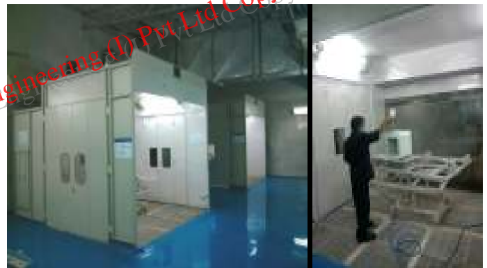
Painting With Paint Booth + Oven + Air Supply Unit & Dust proofing Expertise By Autocoat
