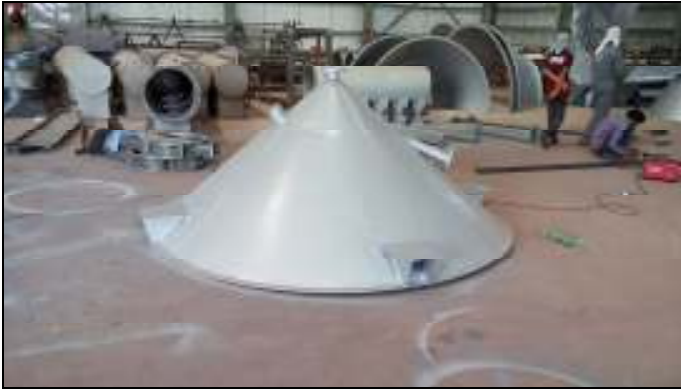
Painting Without Paint Booth Lot of Heavy Paint Dust all Over
