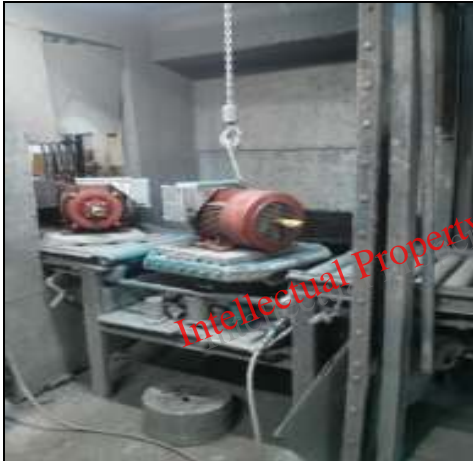
Painting with wrong paint booth unable to meet production
