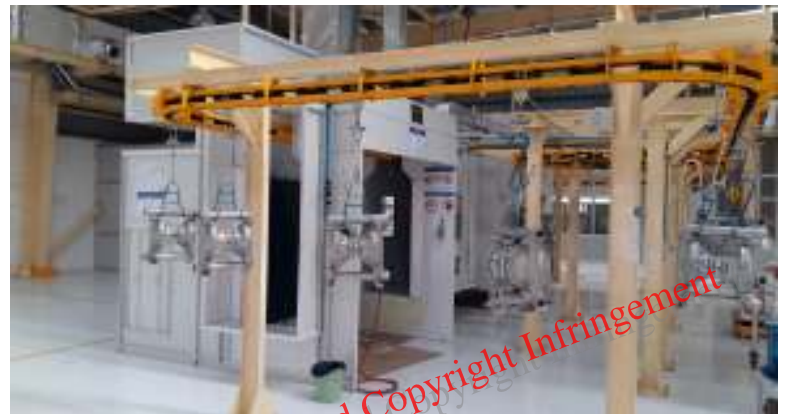
Painting With Paint Booth + Oven + Conveyor + Air Supply Unit & Dust proofing Expertise By Autocoat
