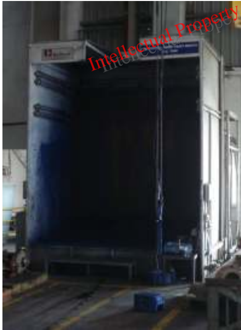
Paint Booth( wrong design) & without material handling
